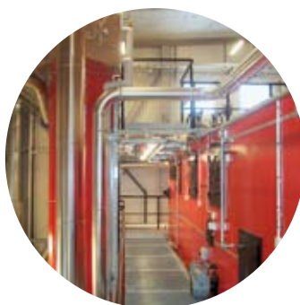
2003: Mora Wastewater Treatment Plant, Sweden 840 tons dry solids per year
